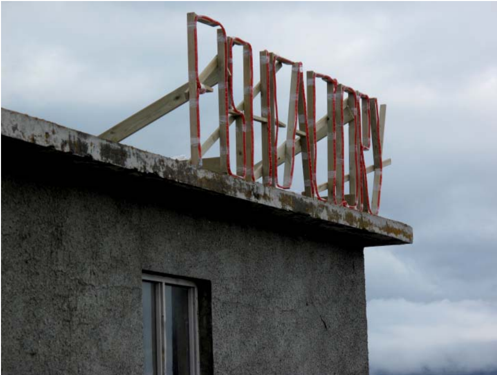
Installation of a lightsign for the exhibition Kvörn at Hyalteri, Iceland, on an abandoned building that is now in use for artexhibitions in northern Iceland. 2009
